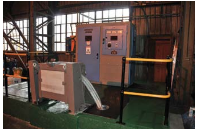
In March the foundry installed a 100 kilogram furnace equipped with an Inductotherm Power-Trak 125-30R power source. This unit forms the heart of the new R&D facility. This furnace also allows the company to perform a specialised service in that Sigma Wear Parts can now offer a quick turnaround time for those urgent one-off castings and low volume castings in non-standard metal such as inconel and barium bronze. The size of this furnace dictates the weight of the casting - a maximum of a 50 kilogram net weight. Sigma Wear Parts will be able to manufacture castings in most metals from this unit
