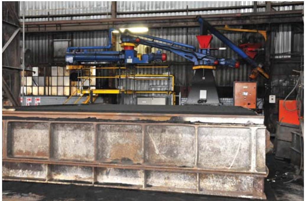
Weir Heavy Bay Foundry installed a new 20 ton an hour continuous mixer supplied by Lauds Foundry Equipment
