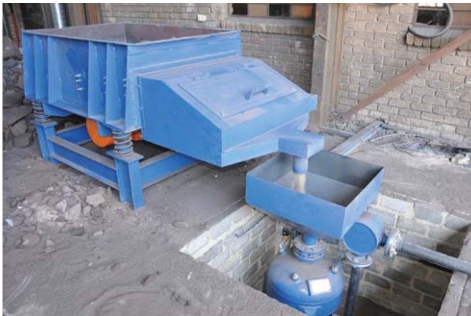
RC Systems were engaged to supply a range of new equipment. This included a 3 ton an hour reclamation system, a shakeout and dust collection unit
